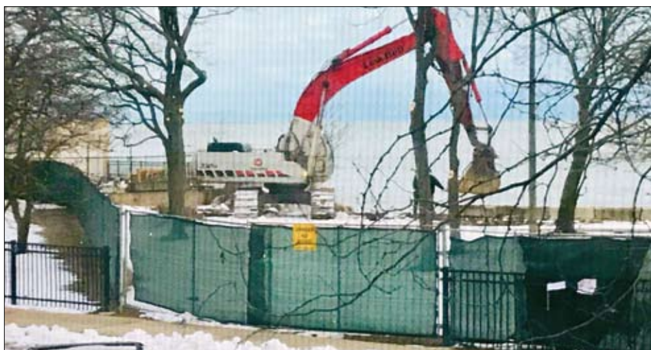
At 7:30 a.m. Monday morning, construction crews at Rogers Beach were “rocking up our last hope for beach access,” said neighbor Reid Hyams, who called what is happening, “The Meigs Field of 2020.” Photo by Reid Hyams
