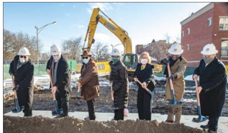
Developers break ground on three-building mixed-income housing project on Chicago's Near North Side.
