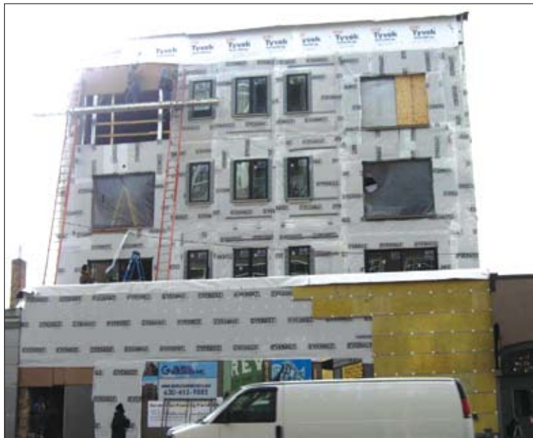
The new four-story Chicago Mosaic School is under construction at 1127 W. Granville. The school aims to increase awareness and appreciation of the ancient art form.
