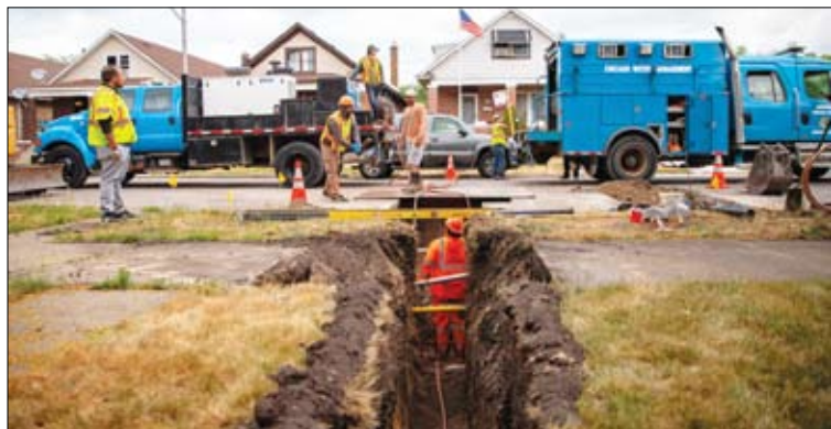
A construction crew completes a lead service line replacement at a Chicago home in June 2023. Courtesy Vanessa Bly/NRDC
