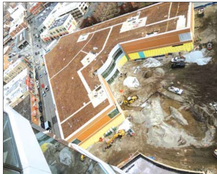
Looking down on the unfinished commercial portion now with halted street to the left.
