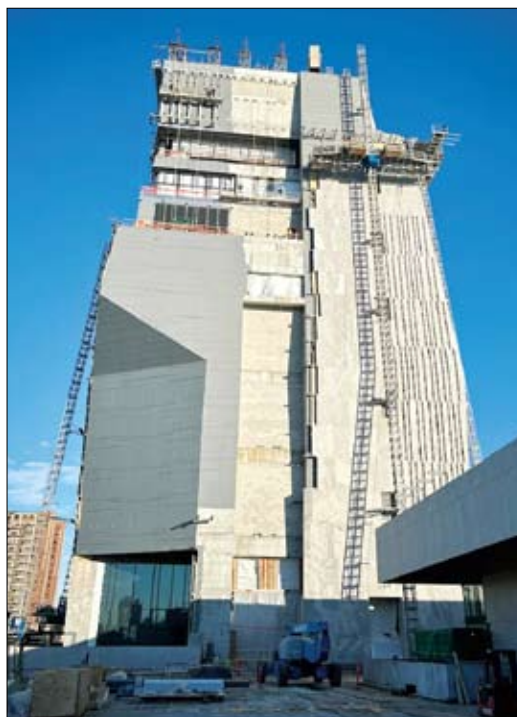
The Obama Presidential Center under construction. Courtesy of The Obama Presidential Center
