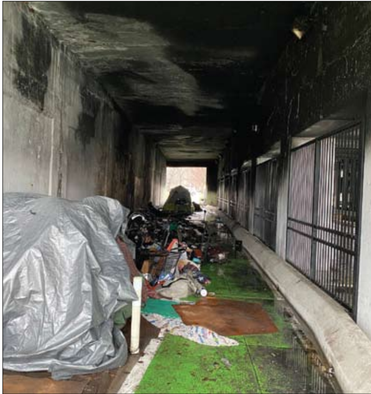
The Lawrence Ave. viaduct under Lake Shore Dr. after a propane tank explosion and fire in 2022. Image courtesy Uptown Update
