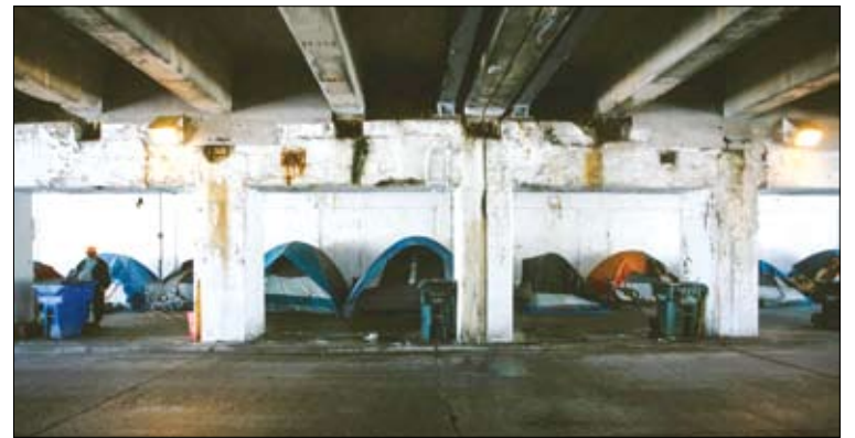
The blockage of all or part of the pedestrian and bike lanes under the viaducts is an ongoing violation of the Americans With Disabilities Act, but the City, State and Park District have chosen not to enforce those laws.
