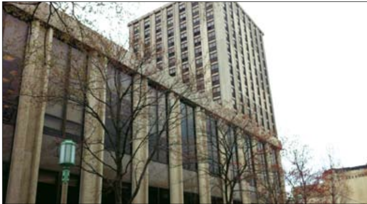
Now under demolition, the Centennial Forum, 1125 W. Loyola Ave., will be closed off until Oct. 9.
