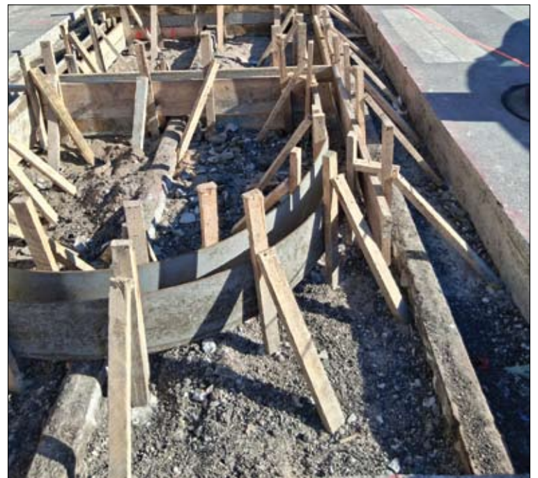
(Top) A one-time streetcar barn still stands at 5837-45 N. Broadway. (Bottom) Old streetcar tracks revealed on Broadway during recent construction of refuge islands.
