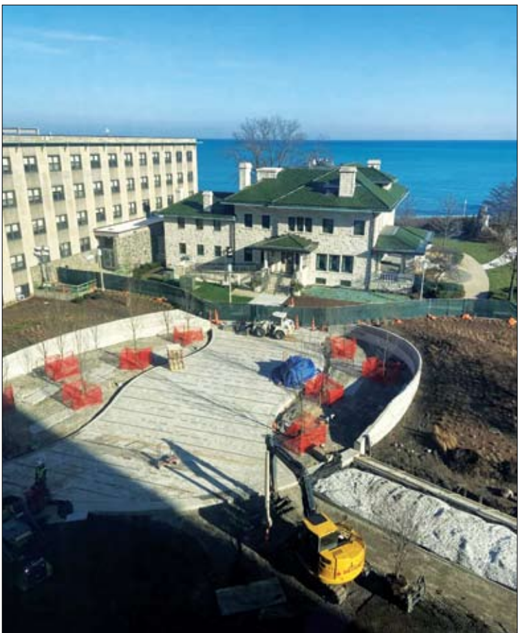
Rev. Stephen Mitten, S.J. said that Loyola's, "Drainage landscaping is a disaster with mulch and dirt flowing right into the drainage sewers, and then they wonder why the building basements flood."
