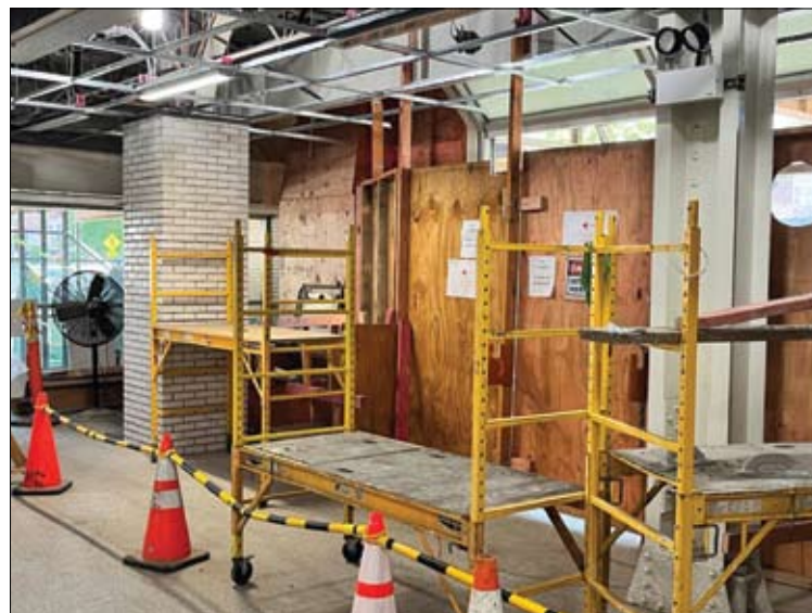
After construction work has been completed, accent lighting will highlight the historic segment of the Berlin Wall that is at the Western Ave. station.
