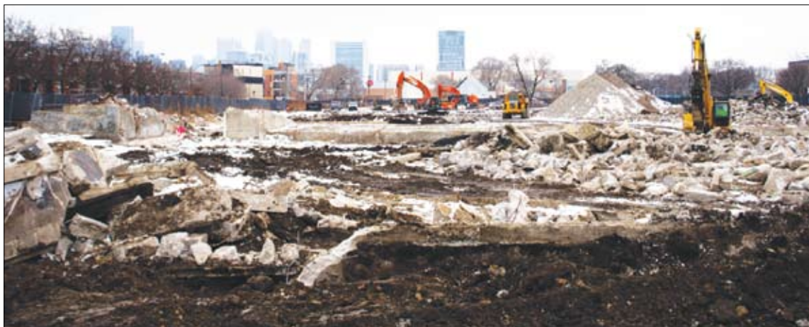
The long-shuttered Near North Career Metropolitan High School was demolished with the help of property tax funds set aside for the redevelopment of the area through a tax increment financing fund. Construction, which is ongoing, is part of the Chicago Housing Authority's plan to redevelop the former site of the Cabrini-Green public housing buildings. Photo by Davon Clark, CatchLight Local
