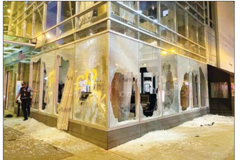
Riot damage to the Wit Hotel at State and Lake streets in the Loop.
