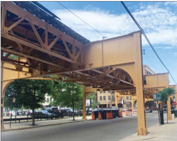
The elevated tracks in the 42nd Ward had not been painted in years and was covered in rust.
