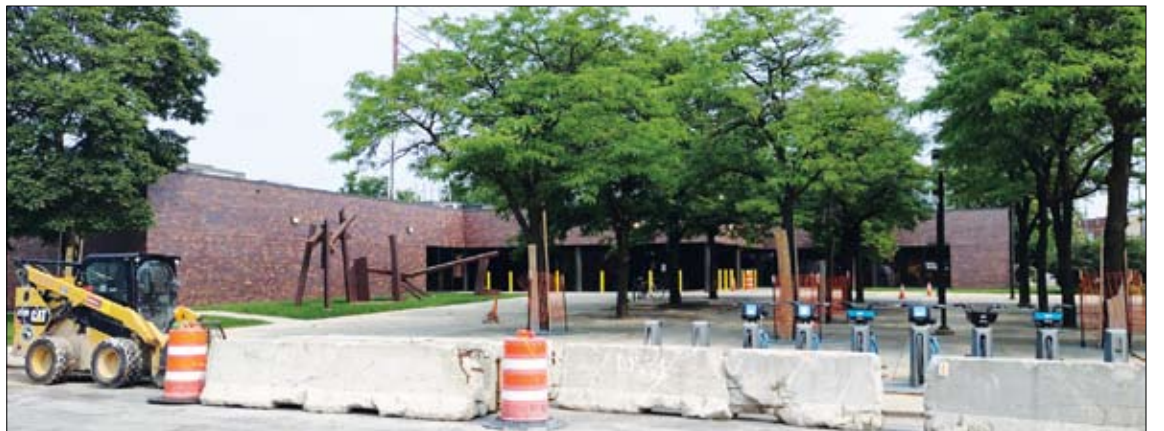
One of the first steps in the Clark St. streetscape project is renovating the courtyard at the Chicago Police Department's 24th District, 6464 N. Clark St.
