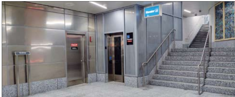
(Top) New turnstiles and fare machines are part of the interior improvements. (Bottom) Elevators and escalators are important accessibility features in the renovated stations.
