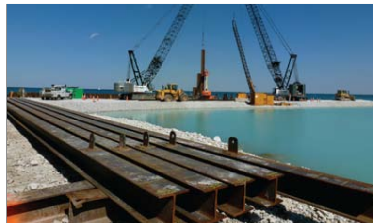
Giant steel poles, or pilings, are pounded 80 feet into the sand and then attached at the visible eyelet to the horizontal sheeting for lateral stability.
