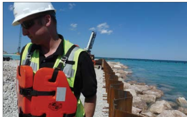
Steven Miskowicz, Senior Project Manager, with the steel sheeting that will encompass the entire job site.
