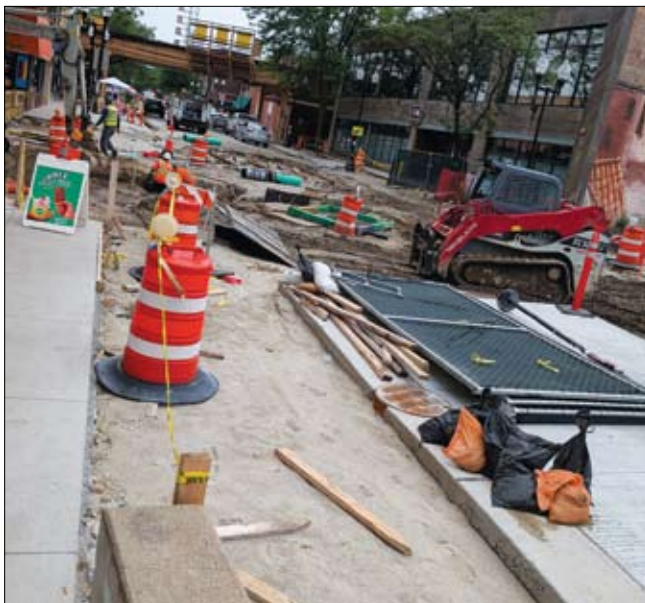
Lincoln Ave. has been blocked off to vehicles for the construction of a privileged biking Greenway on Leland. In an email sent out by Ald. Matt Martin, he did not mention the delays incurred by the ongoing construction projects in Lincoln Square nor the disruptions these have had to the neighborhood’s businesses. He did, however, mention he had spent part of the week with Zac Blanchard, a member of the Baltimore City Council.
