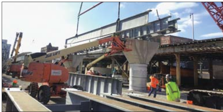
CTA continues to make progress in building the new northbound Red and Purple Line structures. Contractor Walsh-Fluor is building new track structure foundations as well as the new track bed structure.
