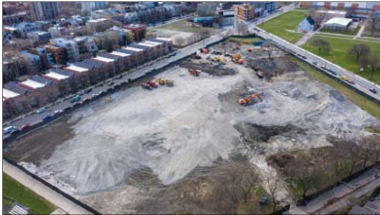
The long-shuttered Near North Career Metropolitan High School was demolished with the help of property tax funds set aside for the redevelopment of the area. Construction, which is ongoing, is part of the Chicago Housing Authority's plan to redevelop the former site of the Cabrini-Green public housing buildings.
