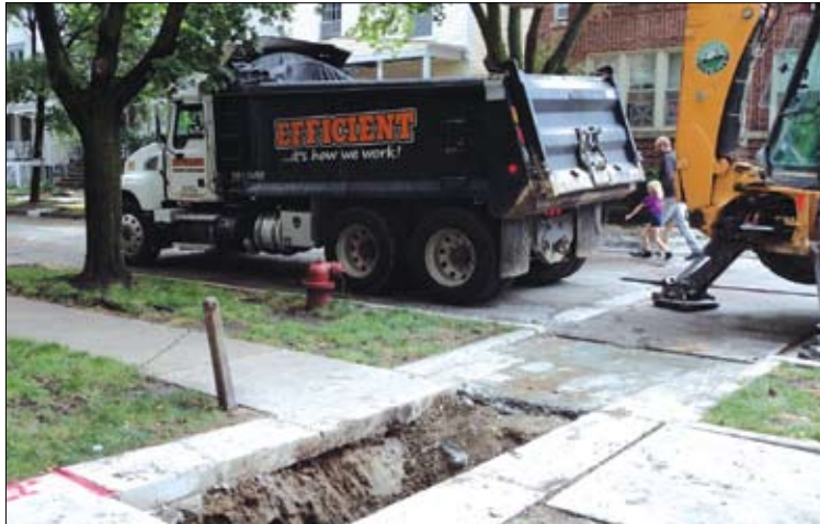
In Edgewater's Rosemont and Glenwood neighborhood, preparations are being made to install the high-speed fiber network for CPS elementary and high schools; 81 schools are expected to be connected by October.
