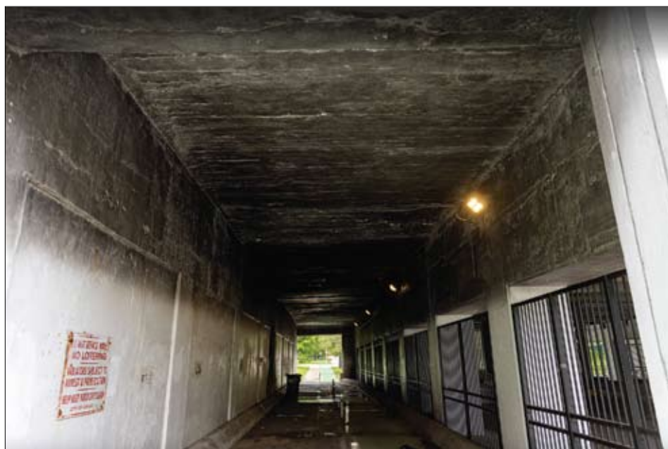
Fires from propane tanks and other flammables have left their mark on the ceiling of the Wilson viaduct of Lake Shore Dr., potentially weakening the structure through spalling (where chunks of concrete break off), cracking (due to thermal expansion), and color changes from extreme heat.
