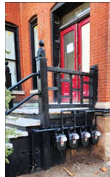
A front porch, railing fence and window at 2420 N. Geneva Terrace have been removed.
