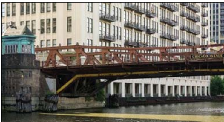
The Chicago Avenue Bridge is scheduled for demolition this month. Photo by James Pillips
