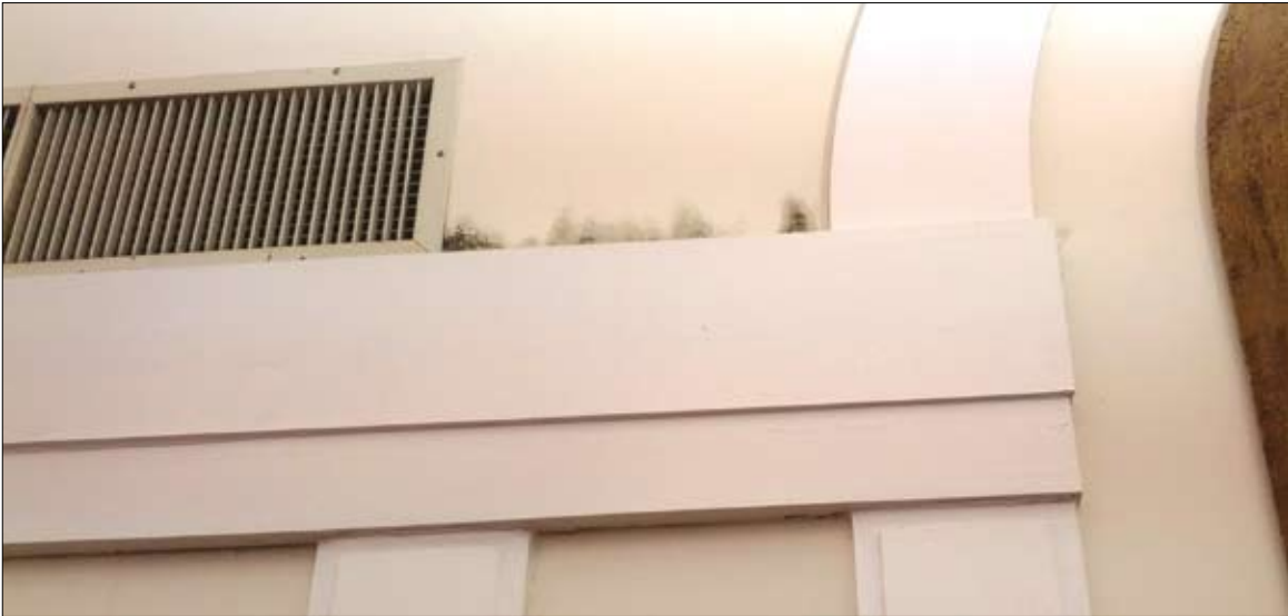
Sharp-eyed library visitors can look at the walls, floors and ceilings throughout the Sulzer Library and see molds that grow openly along seams and corners of the walls and ceilings in the public section of the library. The worst of it may creep down out of sight as it prefers the dark.
