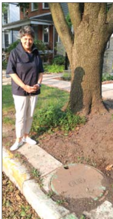
Sally Smith next to the troublesome sewer.
