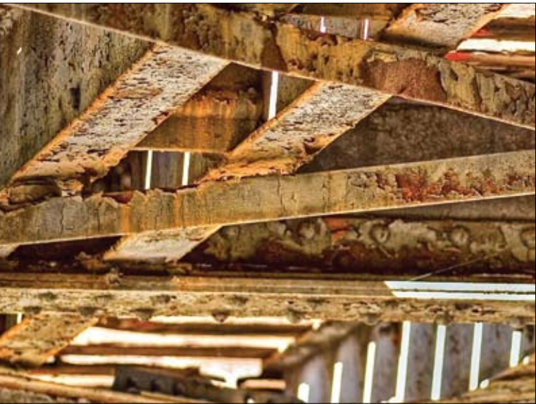
Rust is a menace of corrosion on Chicago's buildings, bridges and pipelines. Photo by Randen Pederson
