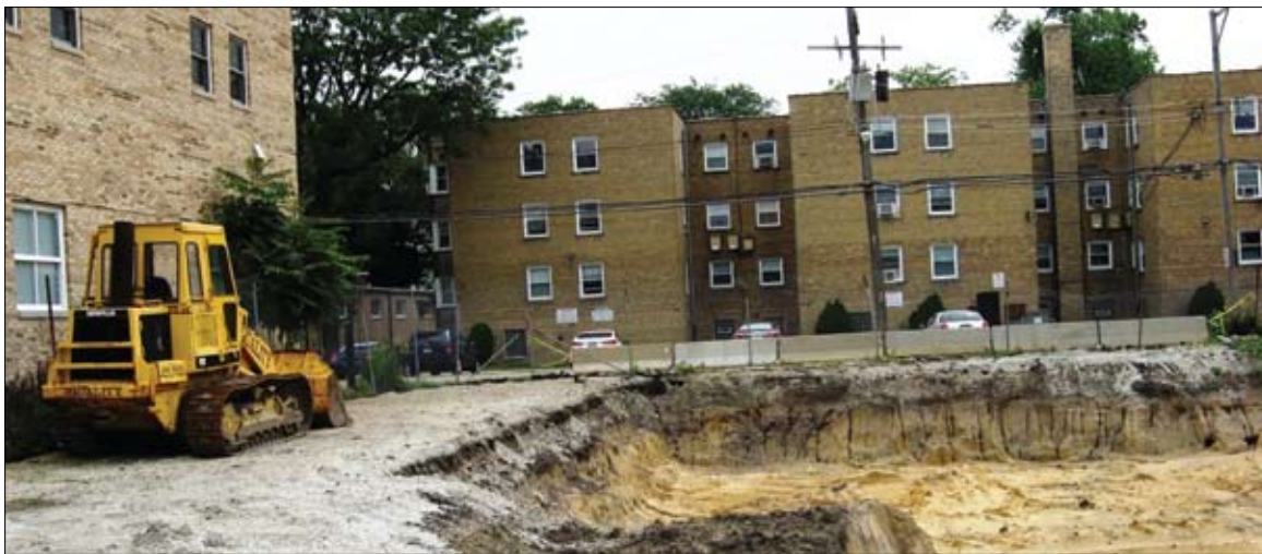
Construction has begun on Tree House's new center that will feature diverse cat suites, calming safe spaces, a veterinary clinic and a Cat Café.
