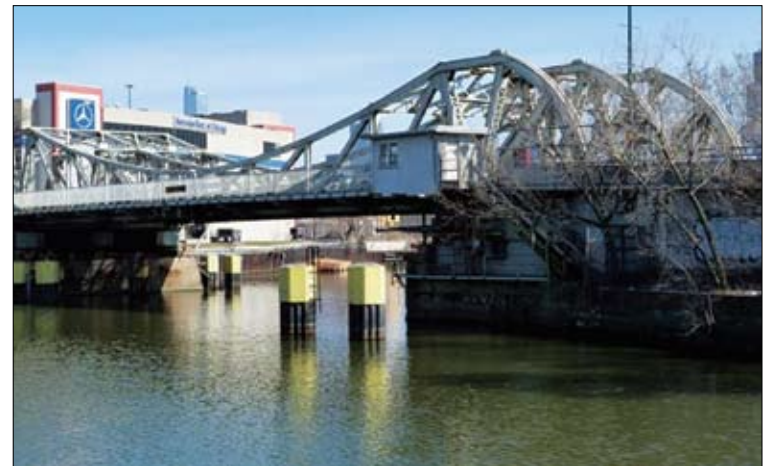
Repair work on the Division Street Bascule Bridge over the North Branch Chicago River began, Jan. 2, and is expected to last until Feb. 9.
