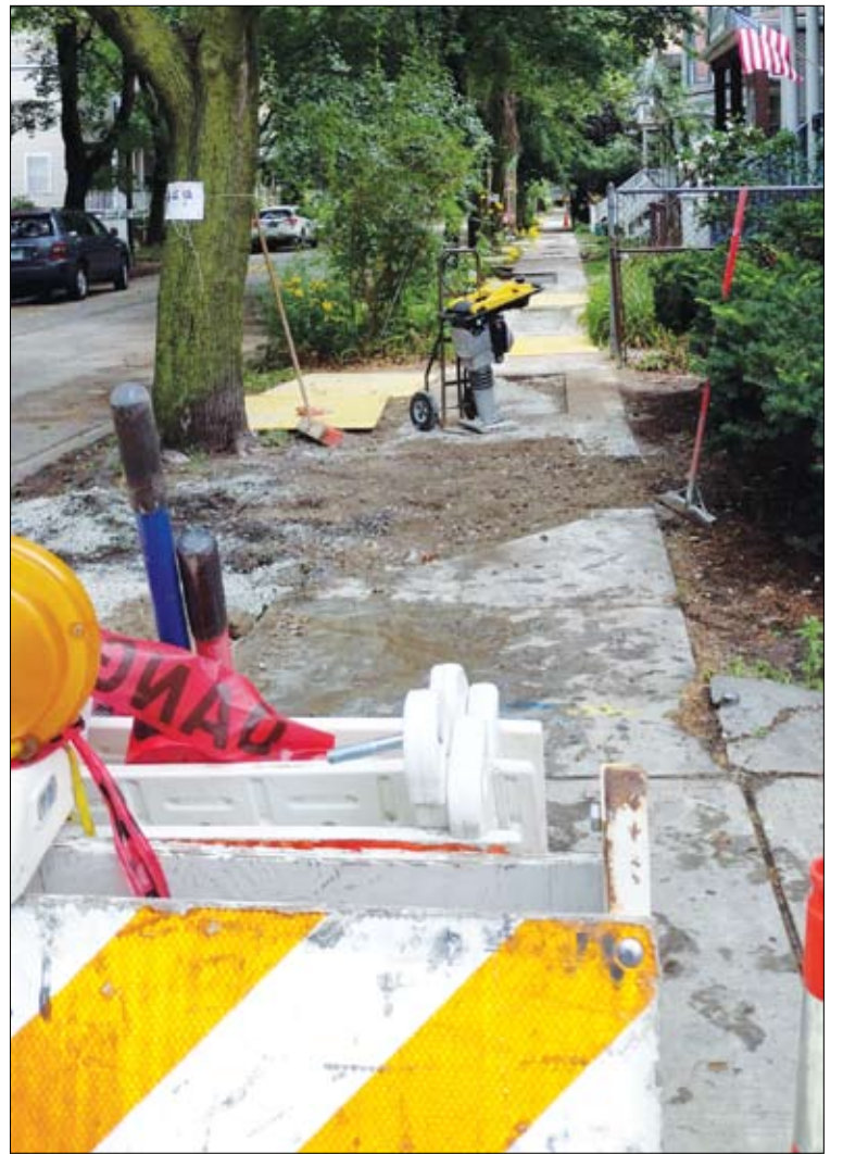
The 1400 block of Highland Ave. is being prepped for the state-of-the-art fiber network to increase internet speeds in Chicago Public Schools. Fiber-optic cables are not subject to electrical interference, which greatly increases the transmission distance. Photo by Joanne Kitsos
