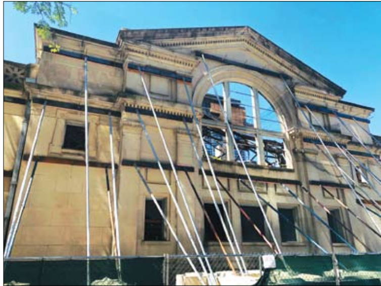
Work has begun in Lincoln Park as developers begin to insert a huge six story building into the middle of what once was The Second Church of Christ Scientist. Already gone to dust and sky, (as is evident in this photo) is the beautiful domed ceiling that was once the architectural centerpiece of this 120 year old Church. Photo by Jim Matusik
